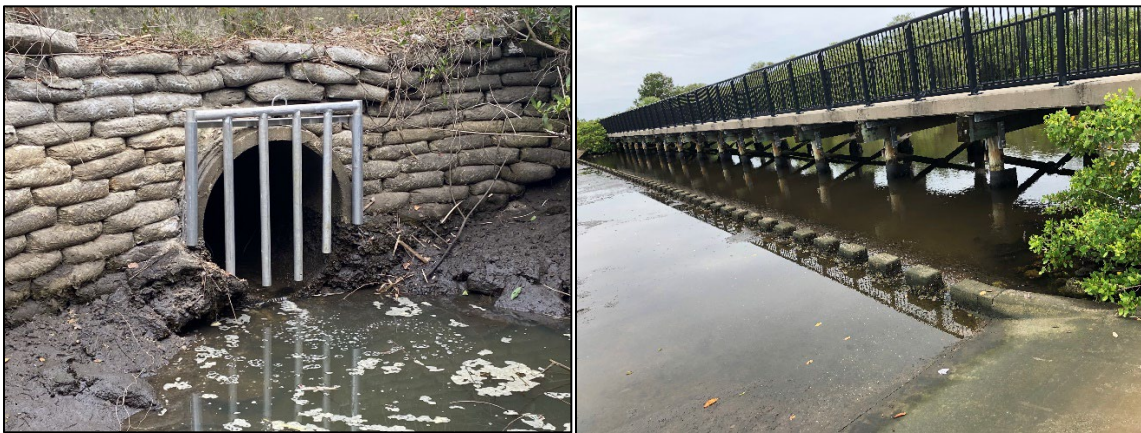
Photo of culvert at Miller's Bayou in Port Richey, Pasco County (left). Photo of spillway near Clam Bayou, St. Petersburg (right).
