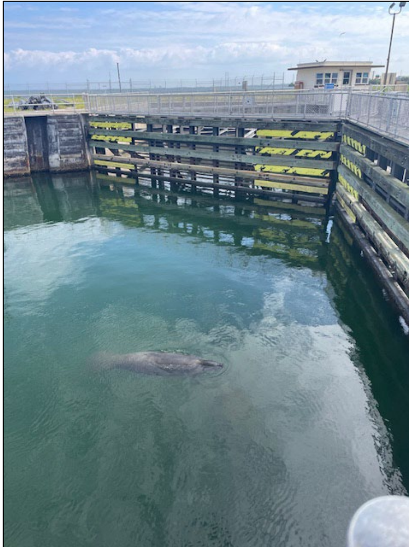
Photo taken during a site visit and agency coordination at Canaveral Lock, one of the structures with a water control structure mortality during the FY 2023-24.
