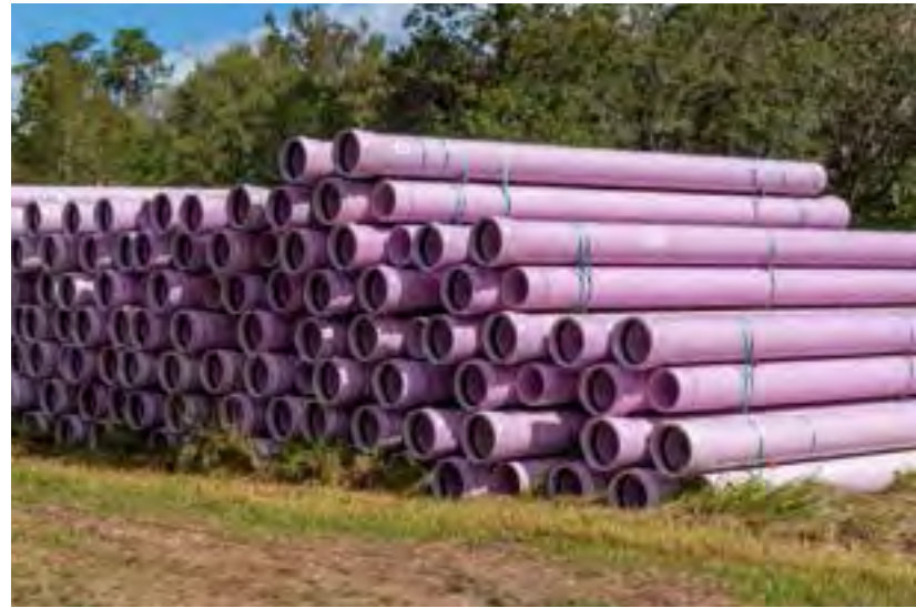
Reclaimed water pipes waiting to be installed.
