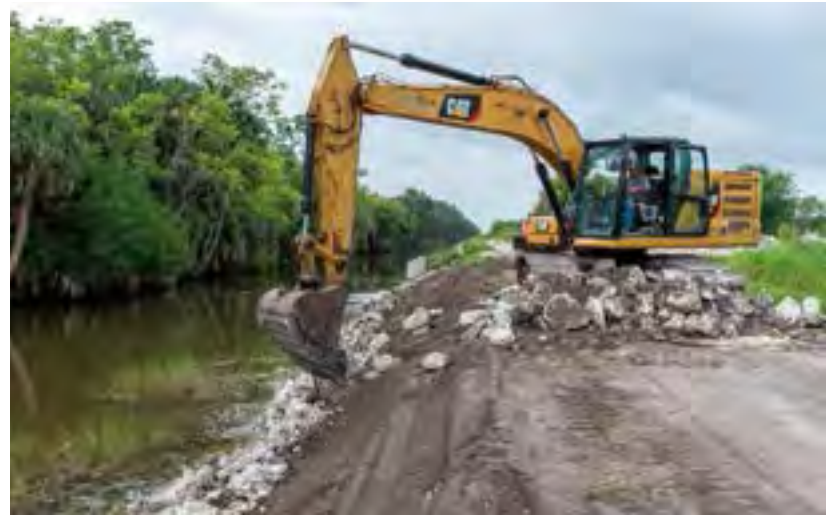
Regrading the levee slopes along the Lake Apopka Wildlife Drive (top). Stabilizing the levee on the Apopka-Beauclair Canal (bottom).
