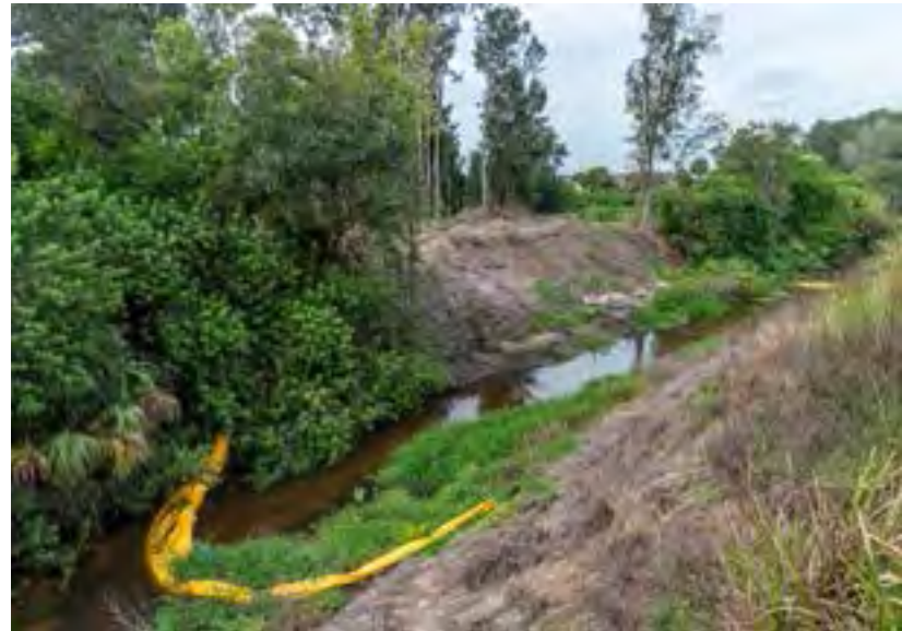
Turbidity curtain in the M-1 canal before construction of a water control structure.
