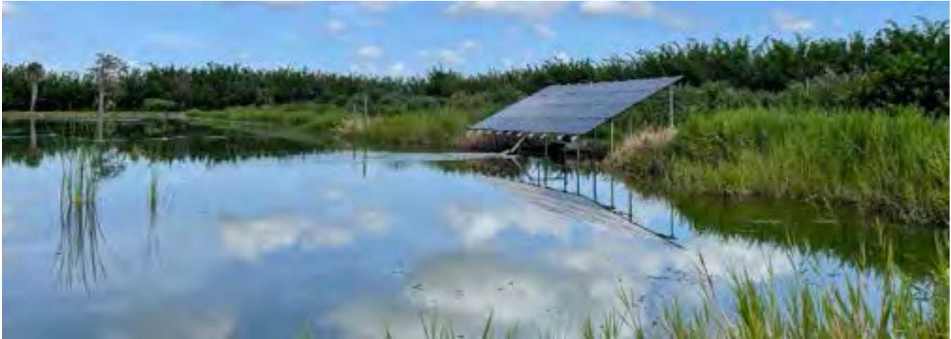
Solar panels power pumps in a surface water conversion cost-share project at Hammond Groves in Indian River County.
