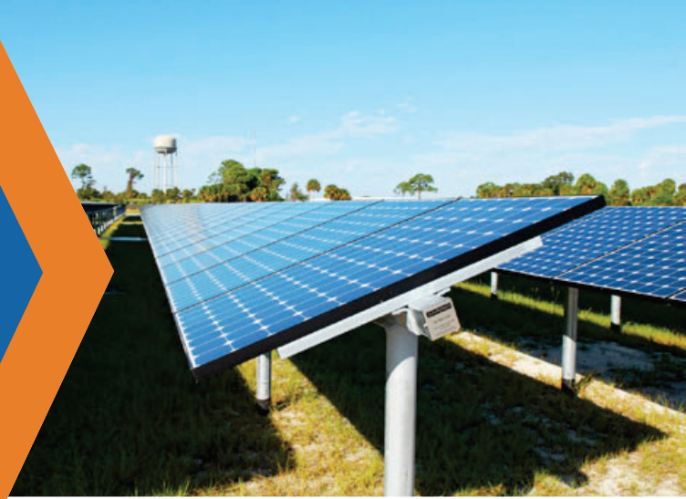
NASA's first large-scale solar power generation facility at Kennedy Space Center. Image credit: NASA.
