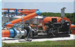
FLM, Inc. Pump Station and Filters
