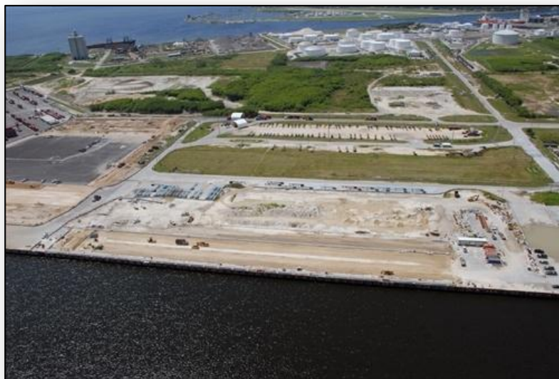
Development of a container cargo terminal facility on Hookers Point at the Port of Tampa.
