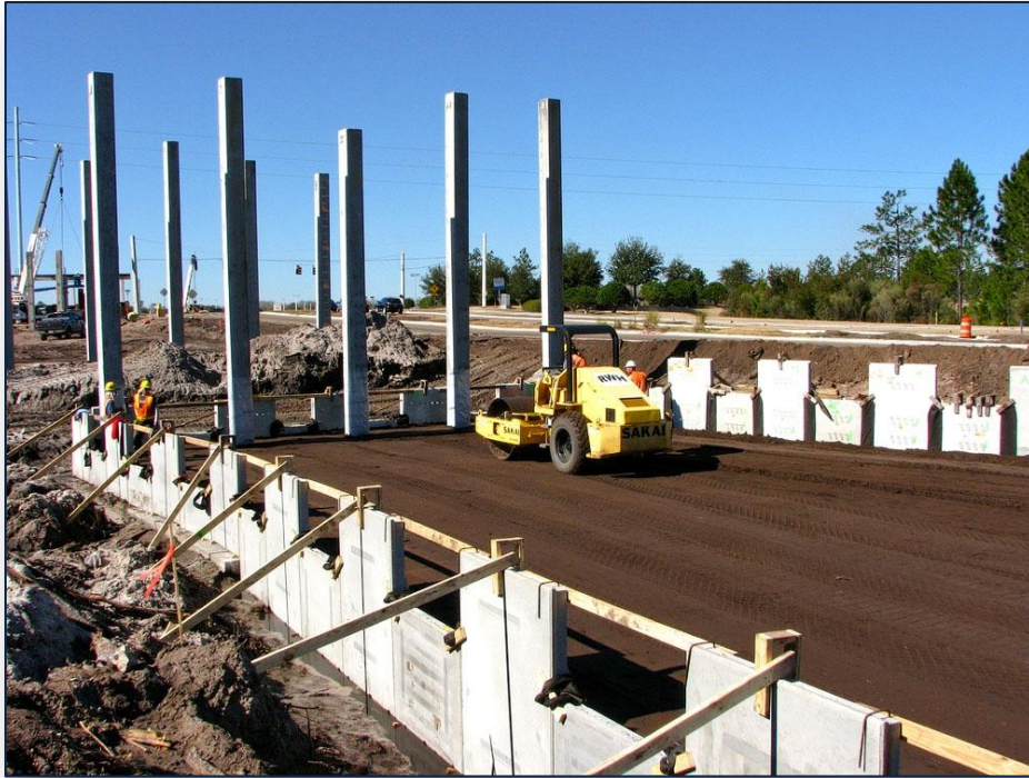
New overpass going up over Branan Field Chaffee Road (SR 23) in Clay County.
