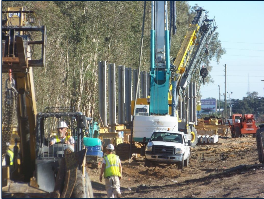
Installation of pilings for sound barrier wall along US 27 in Polk County.
