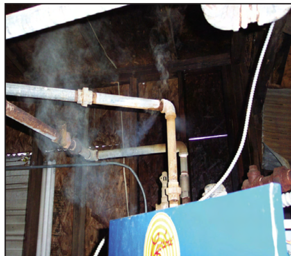
High pressure steam boiler.
