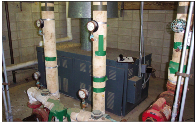
Hot water heating boiler. The live steam blowing from the pictured high pressure steam boiler is less subtle.
