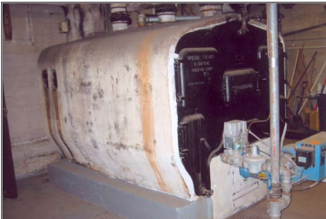
Boiler Located in Pinellas County
