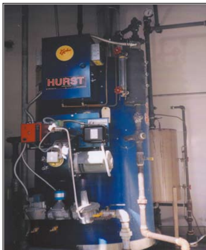
Heating Boiler Installed in Hotel
