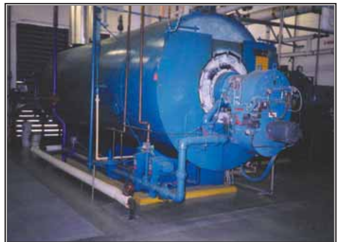
Vertical Boiler Installed in Dry Cleaner
