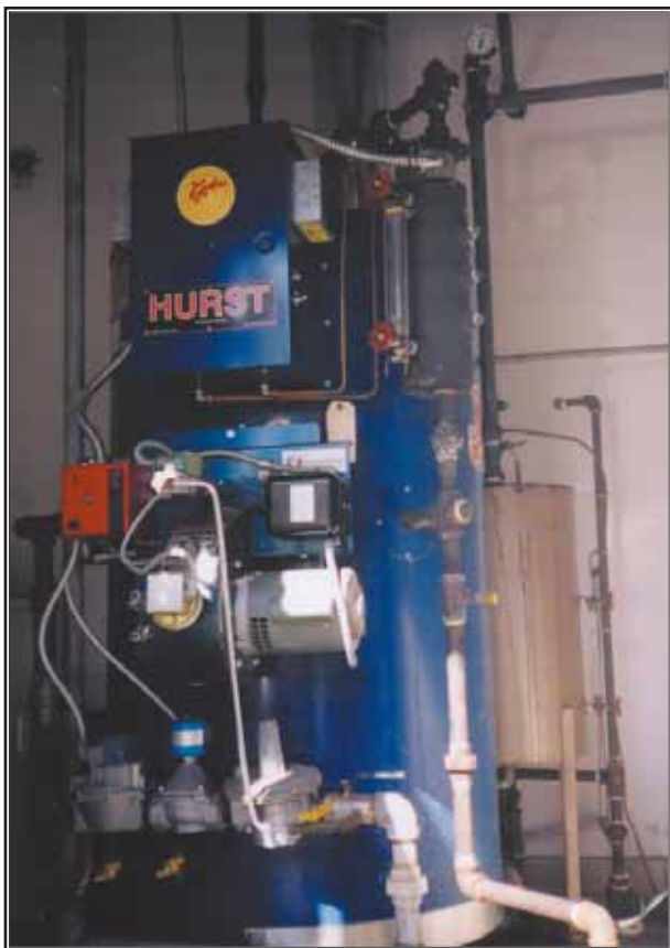
Heating Boiler Installed in Hotel
