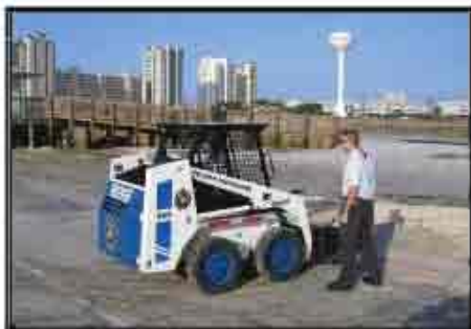
Clint Croft (Bobcat Operator) and Lt. Steadman responding to a mission tasked from State Emergency Operations Center in Navarre Beach Florida.
