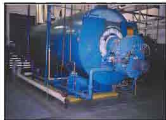
Vertical Boiler Installed in Dry Cleaner
