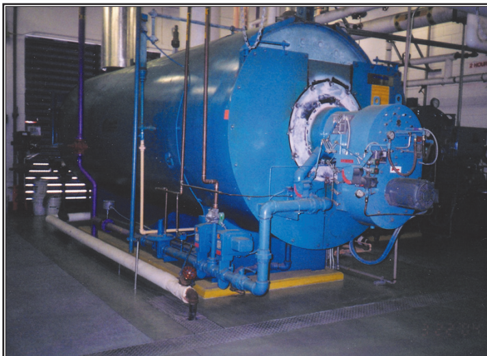
Typical boiler used in a hotel
