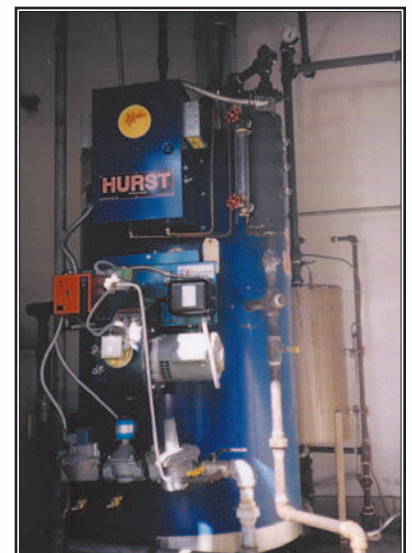
Typical boiler used by a dry cleaner
