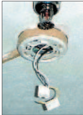
Smoke detector missing
