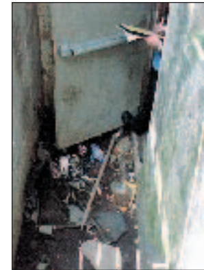
Keep clutter out of exit door pathway
