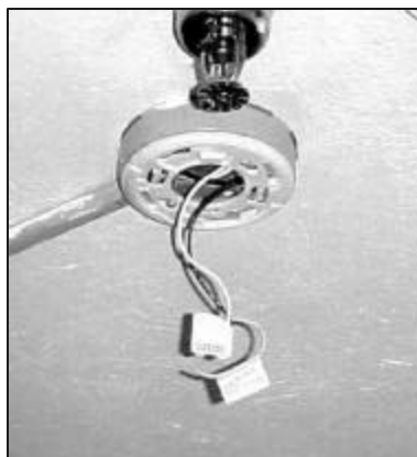
Smoke detector missing
