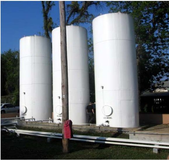
Above Ground Petroleum Storage Tanks
