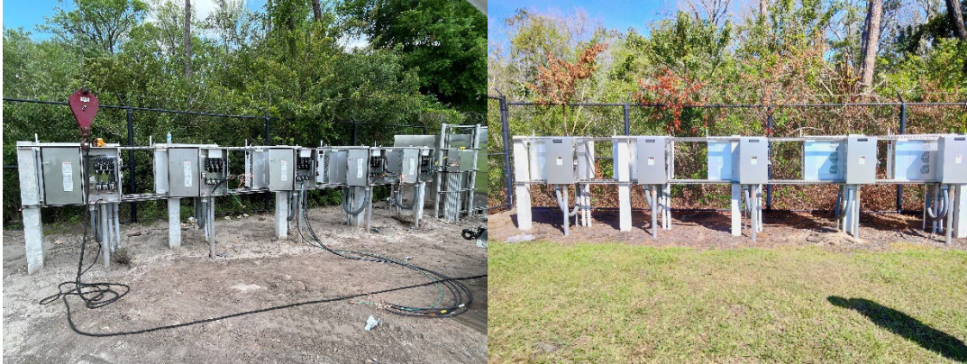
Above photos are pre- and post-install of AC disconnect switches on an existing inverter rack at the Regional Water Reclamation facility located in the City of Altamonte Springs, Florida.
