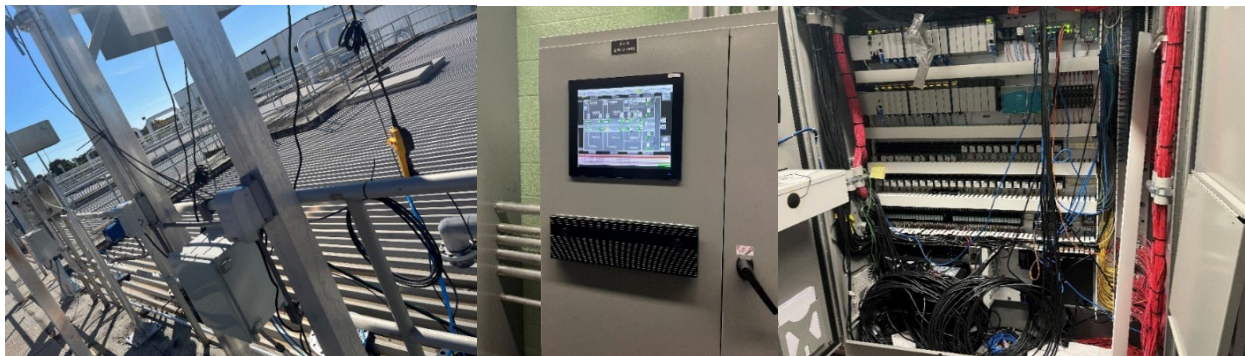
Above photos show the new aeration system for the South Central Regional Wastewater Treatment Plant and Disposal Board.
