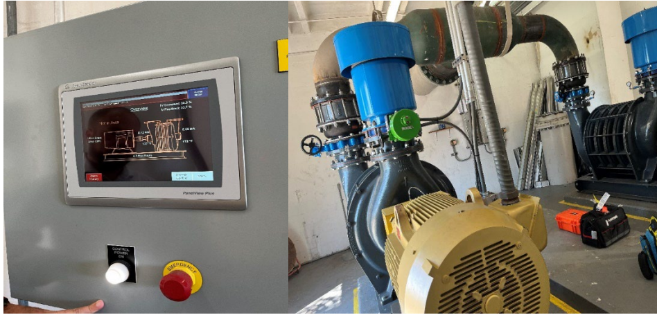
Above photos show the new blower system at Coral Springs Improvement District's Wastewater Treatment Plant.
