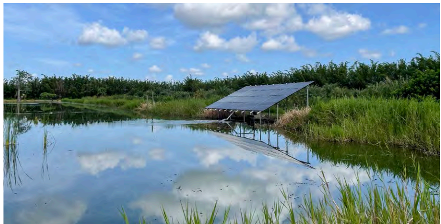
Solar panels power pumps in a surface water conversion cost-share project at Hammond Groves in Indian River County.
