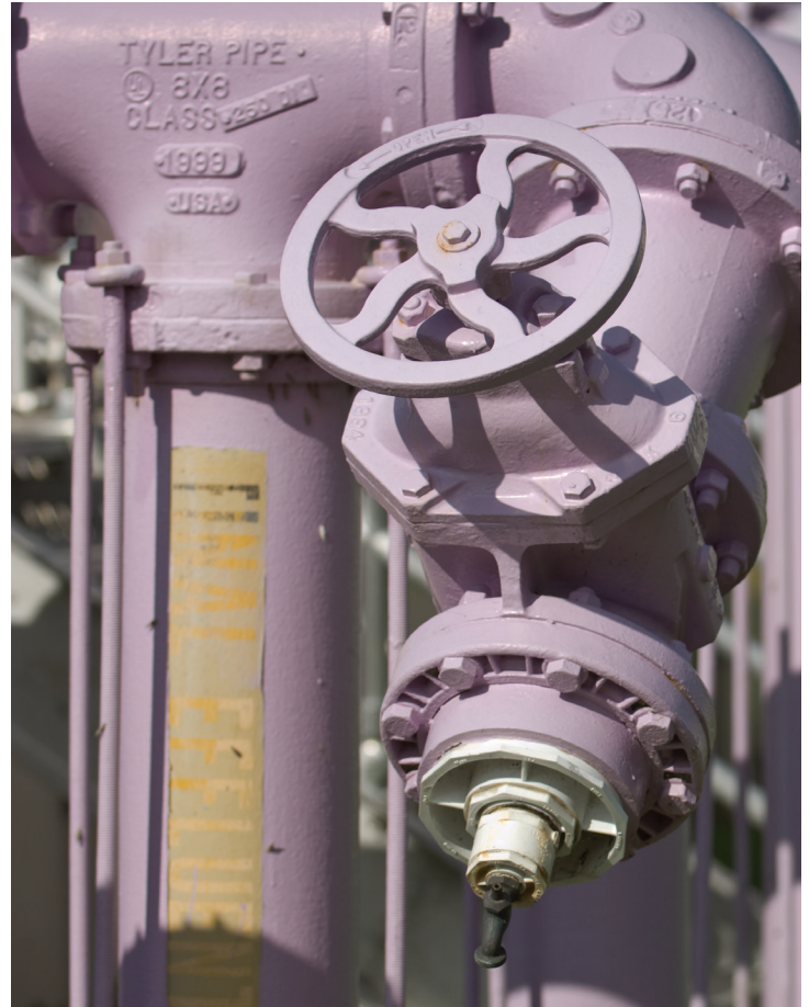
Water Reuse Purple Pipes
