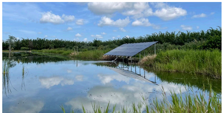
Solar panels power pumps in a surface water conversion cost-share project at Hammond Groves in Indian River County.
