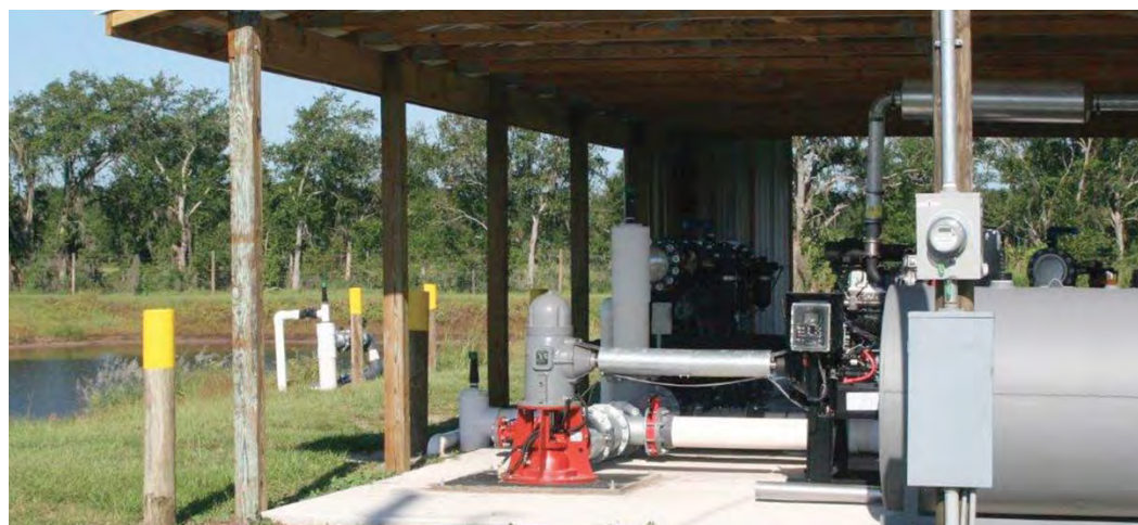
Surface water pump station at Windmill Farms, Hardee County.
