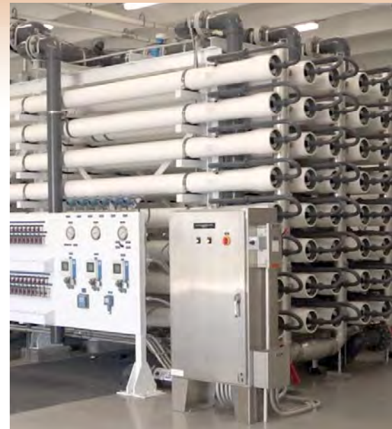
Punta Gorda Reverse Osmosis Water Treatment Facility.
