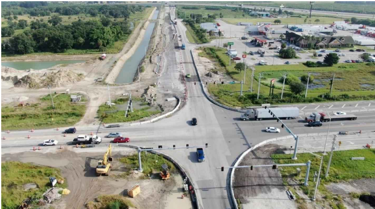
Kings Highway (State Road 713) from South of State Road 70 to North of the I-95 Overpass (District 4)
