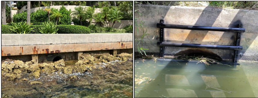
Photo of culvert and living shoreline at Brickell Key in Biscayne Bay, Miami-Dade County (left). Photo of grated culvert in Cape Canaveral, Brevard County (right).
