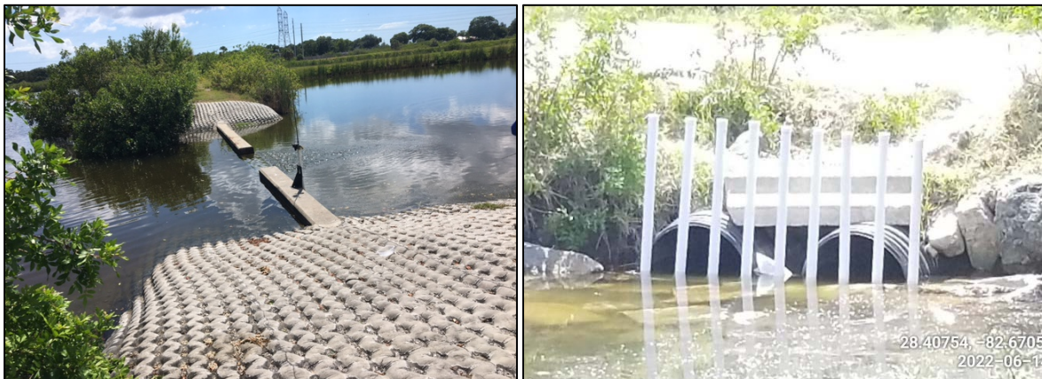
Photo of weir at Mobbly Bayou Wilderness Preserve in Oldsmar, Pinellas County (left). Photo of grated culvert in Sunwest Park, Pasco County (right).
