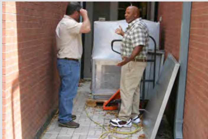
Maintenance Superintendent, Lynn Lee (right) coordinating air handler replacement and installation with Cook Brothers Inc. liaison Jason Layerd (left) (sub-contractor to the Department of Management Services)
