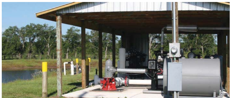
Surface water pump station at Windmill Farms, Hardee County.
