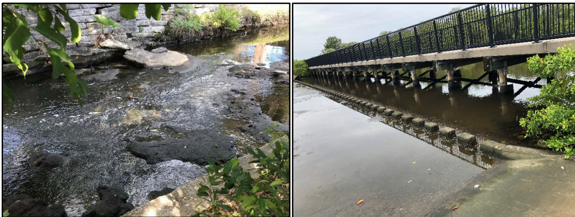
Photo of weir at McKay Creek in Largo, Pinellas County (left). Photo of concrete spillway in St. Petersburg, Pinellas County (right).
