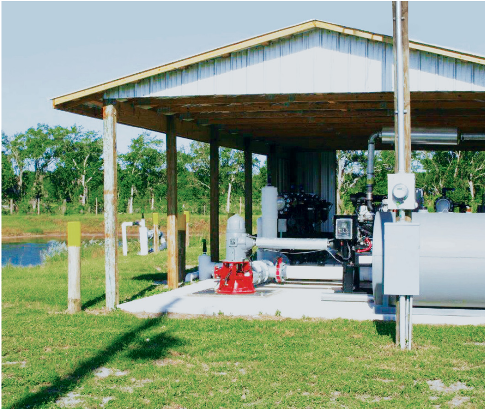
Surface water pump station at Windmill Farms, Hardee County.
