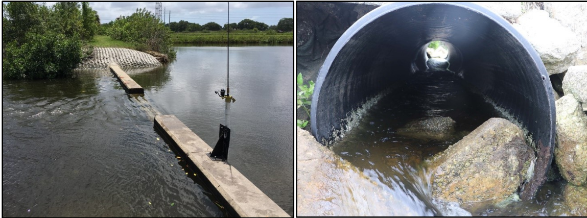
Photo of weir at retention pond in Oldsmar, Pinellas County (left). Photo of a stormwater culvert in Hudson, Pasco County (right).
