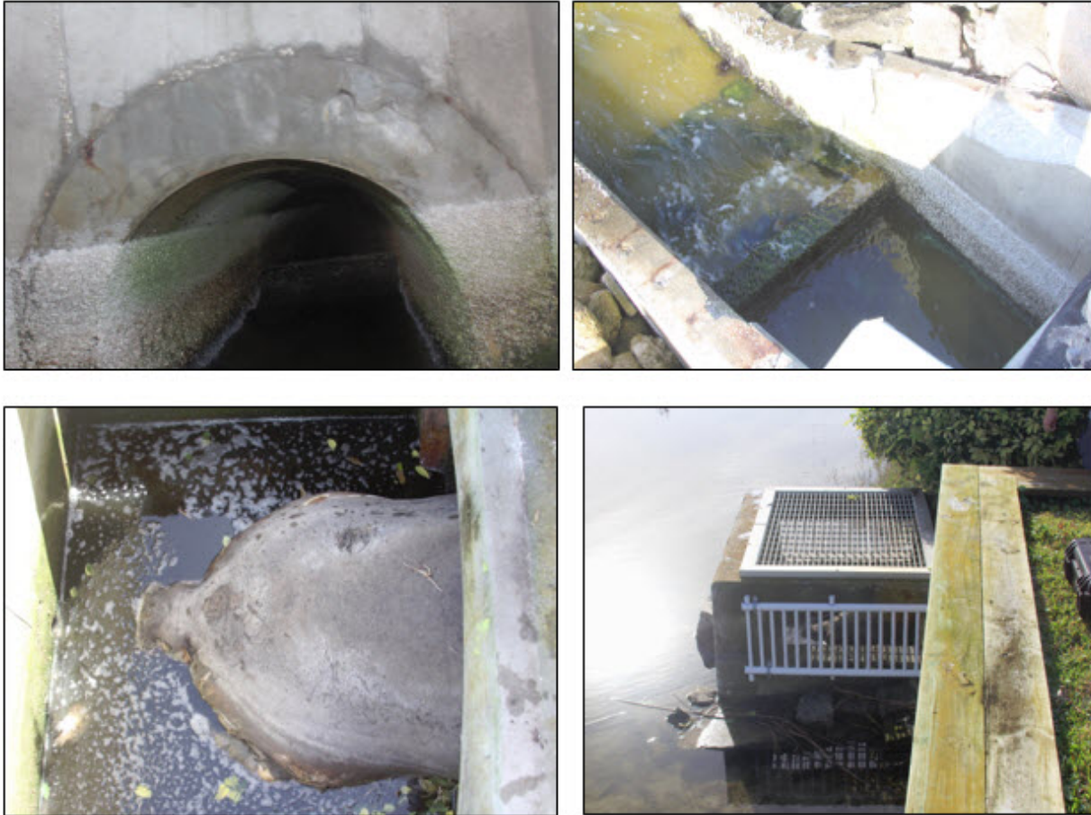
Photos of manatee entrapment incident in a stormwater culvert in the Banana River, Cocoa Beach, Brevard County.
