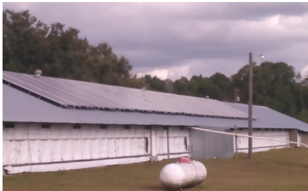
Poultry farm with PV installed
