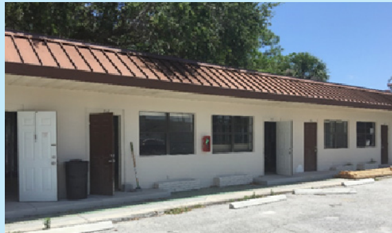
In Indian River County, Camp Haven is renovating an abandoned motel to create efficiency apartments for men moving out of homelessness, thanks to the Treasure Coast Continuum of Care Challenge Grant.
