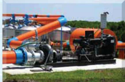
FLM, Inc. Pump Station and Filters
