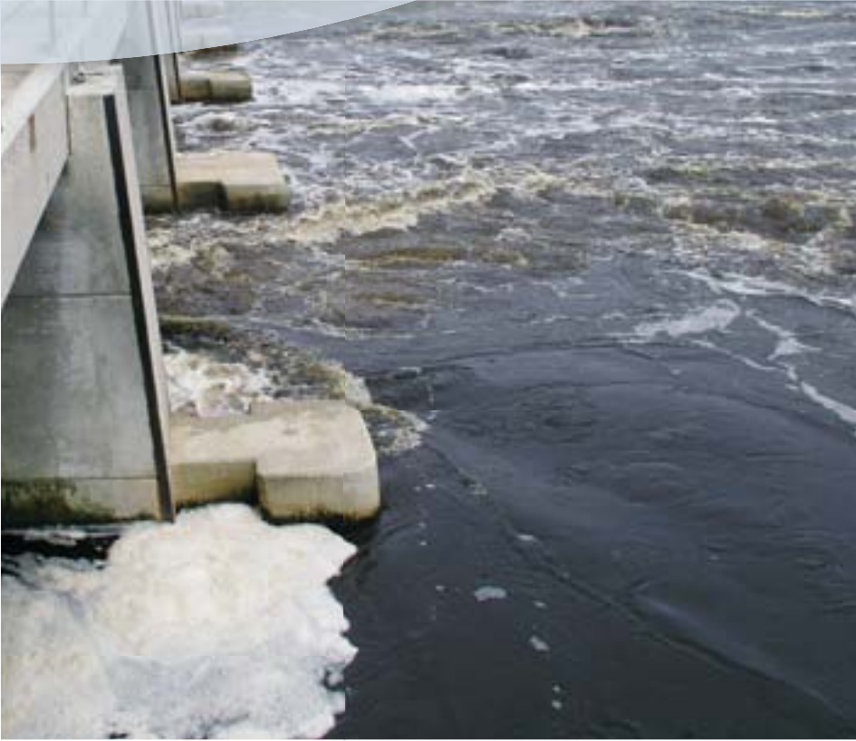
Floodwaters bypass Temple Terrace and Tampa through a structure on the Tampa Bypass Canal.
