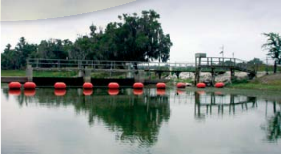
Modification of the structure at Lake Hancock's outfall to Saddle Creek will be key to the Upper Peace River Watershed Restoration initiative, modifying the level of Lake Hancock.
