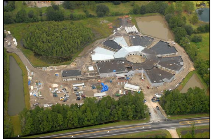
Clyde E. Lassen State Veterans' Nursing Home, Under construction in St. Augustine
