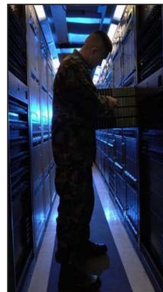
Commission staff evaluates the quality of service provided by telecommunications companies and conducts periodic on-site inspections of telecommunications facilities.
