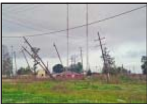
Local exchange telecommunications companies have filed requests for recovery of storm related costs.
