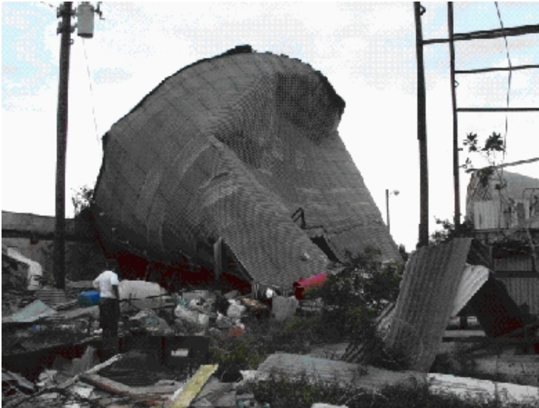
State Owned Property Destroyed by Hurricane Wilma in Hendry County
