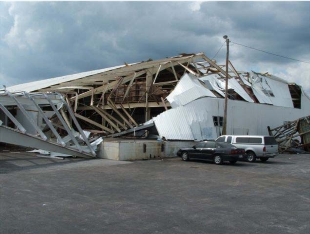
State Owned Property Destroyed by Hurricane Charley in Desoto County
