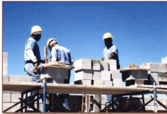
Laying Brick - Sumter Work Camp inmates working at the Citrus County Maximum Risk Facility.
