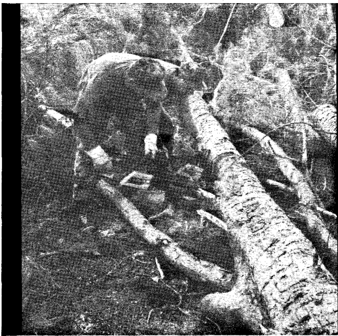
Members of the 202nd RED HORSE Civil Engineering Squadron work to remove debris in the aftermath of Hurricane Andrew.
