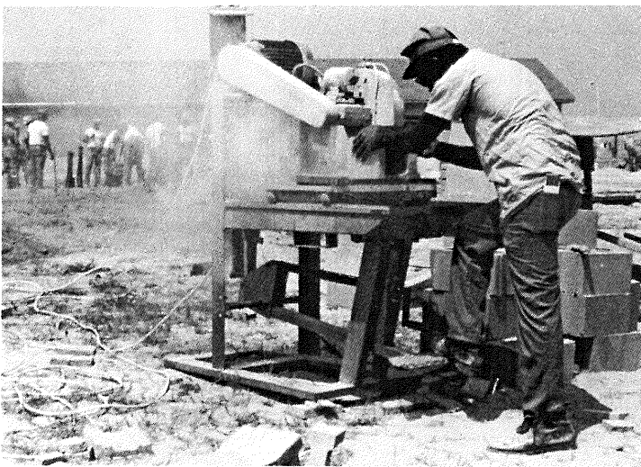
Inmate using masonry saw to shape concrete blocks to the correct size at Walton C.I.
