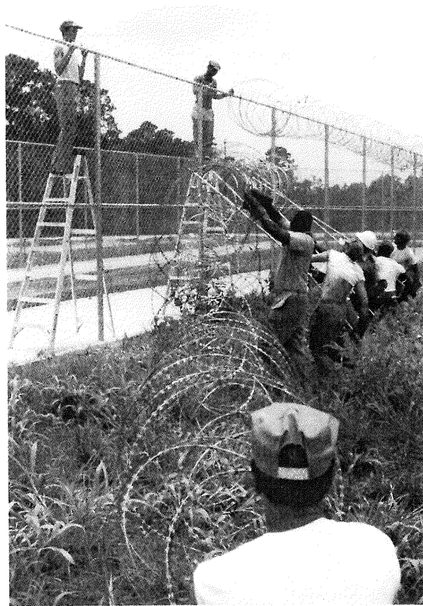
Inmates labor to erect and secure razor ribbon on the perimeter fences at newly constructed Madison C.I.
