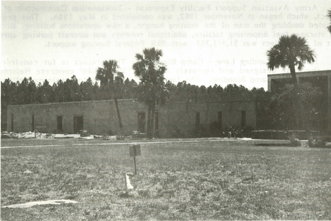
Construction in process at Jacksonville ANG base. Expansion of Operations Building, adding 24,000 square feet
