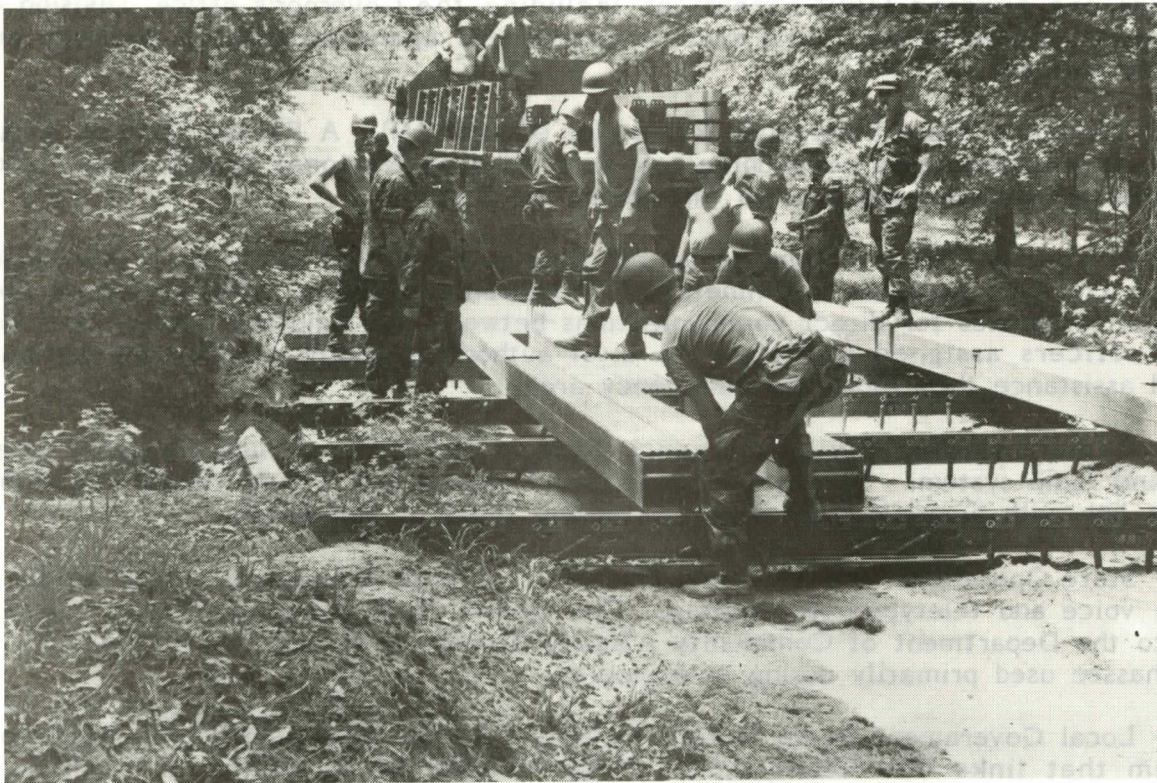
Construction of a temporary bridge over a "wash out" is performed by one of Florida's engineer units. These units are available to Florida counties during disasters
